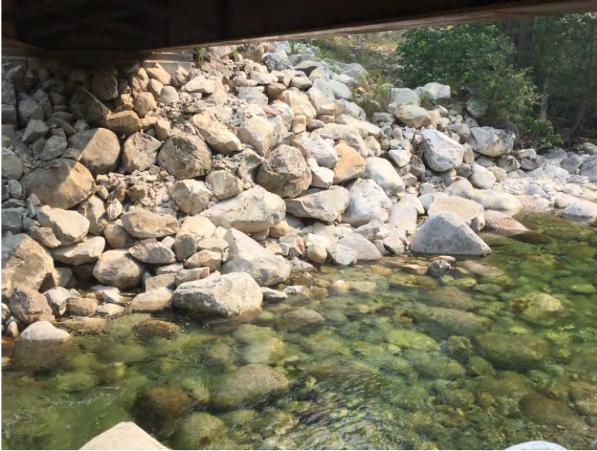
Downstream left bank riprap scour
