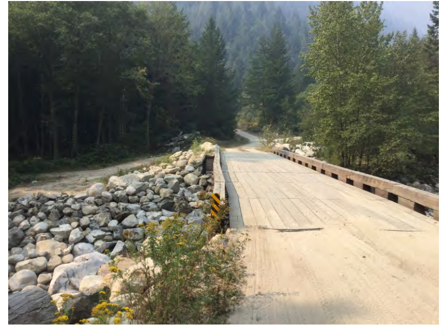
Deck panels misaligned
