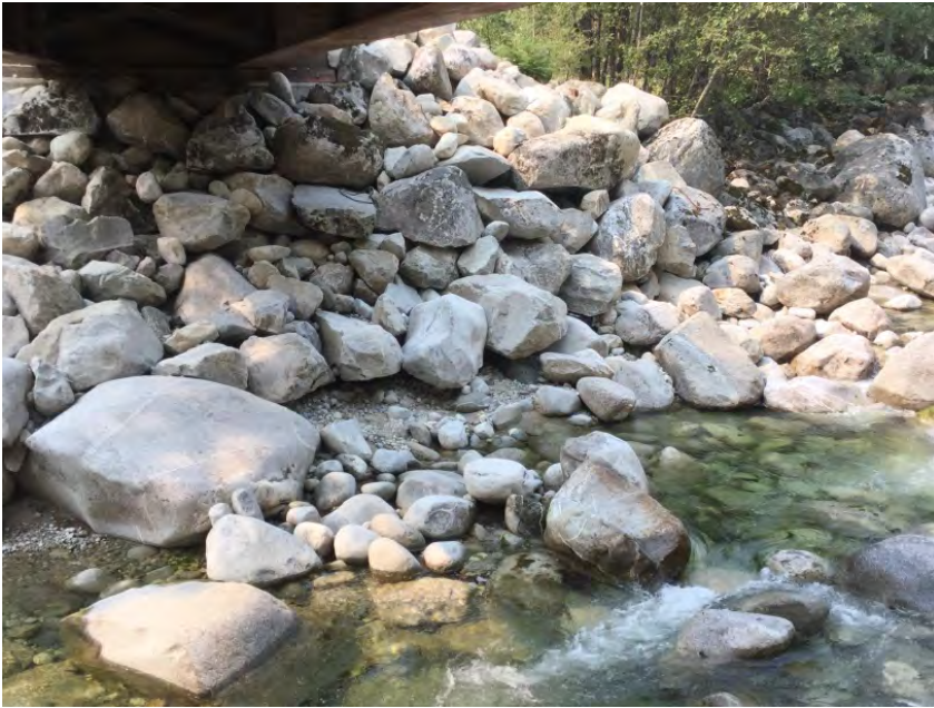
Upstream right bank riprap scour
